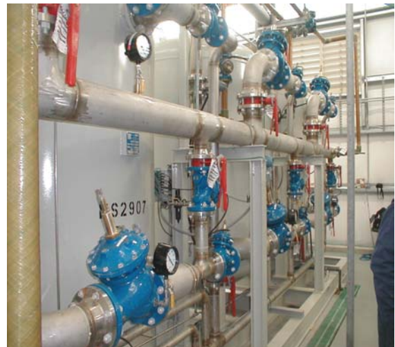
Figure 1: The ASME coded Softener tanks and SS face piping.
