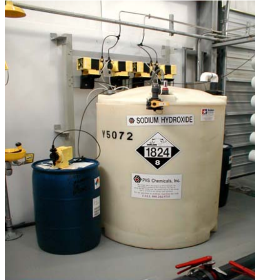
Figure 10: Chemical injection was designed for automated operation and spill containment.
