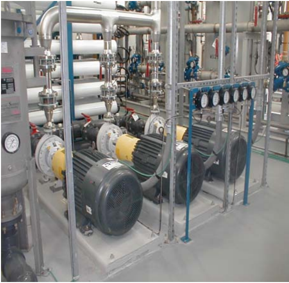
Figure 9: Three feed water pumps were provided with 100% redundancy for operation assurance. Equipment layout was developed to provide safe access for operations, reducing space requirements.
