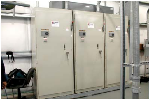
Figure 5: Soft starter panels, soft starters were used to reduce starting load of 150 hp motors.
