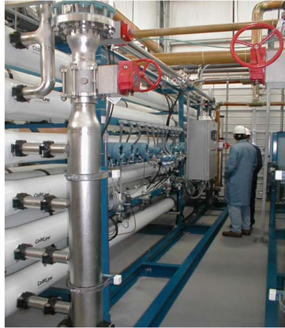
Figure 3: RO Unit, showing the SS feed header, membranes Housings and instruments installed
