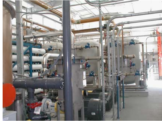
Figure 6: Chemical cleaning system was provided for the RO unit, FRP piping was used for interconnections of equipment.
