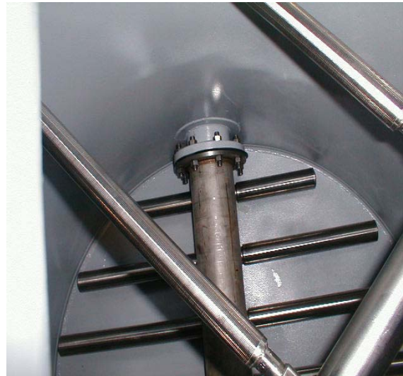
Figure 7: The internal SS headers of softeners were designed to operate at maximum flow rate with a low pressure drop.
