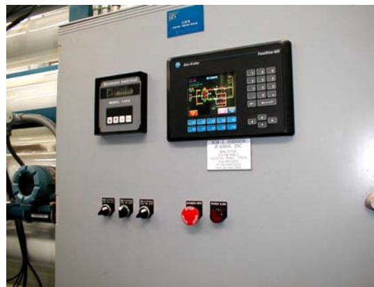
Figure 4: PLC Panel has graphical screens
